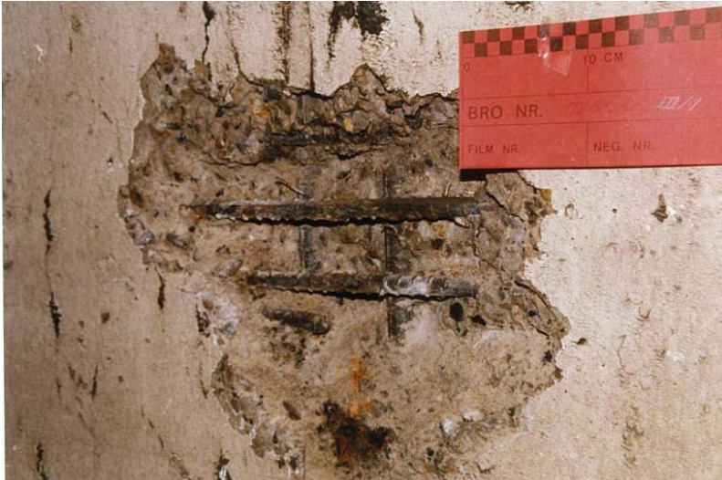
Figure 4.5-1 Reinforcement corrosion from inspection in 1988.
