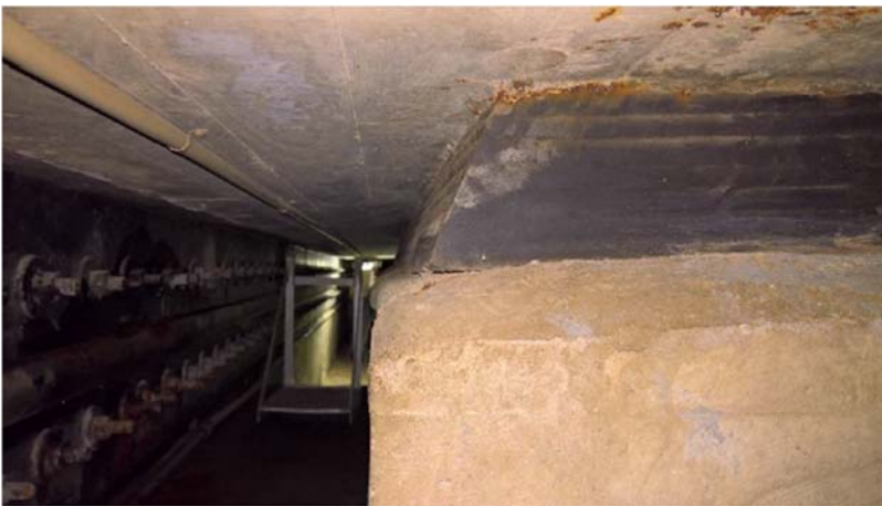
Figure 4.1-3 Elastomeric bearing at the northern portal building.
