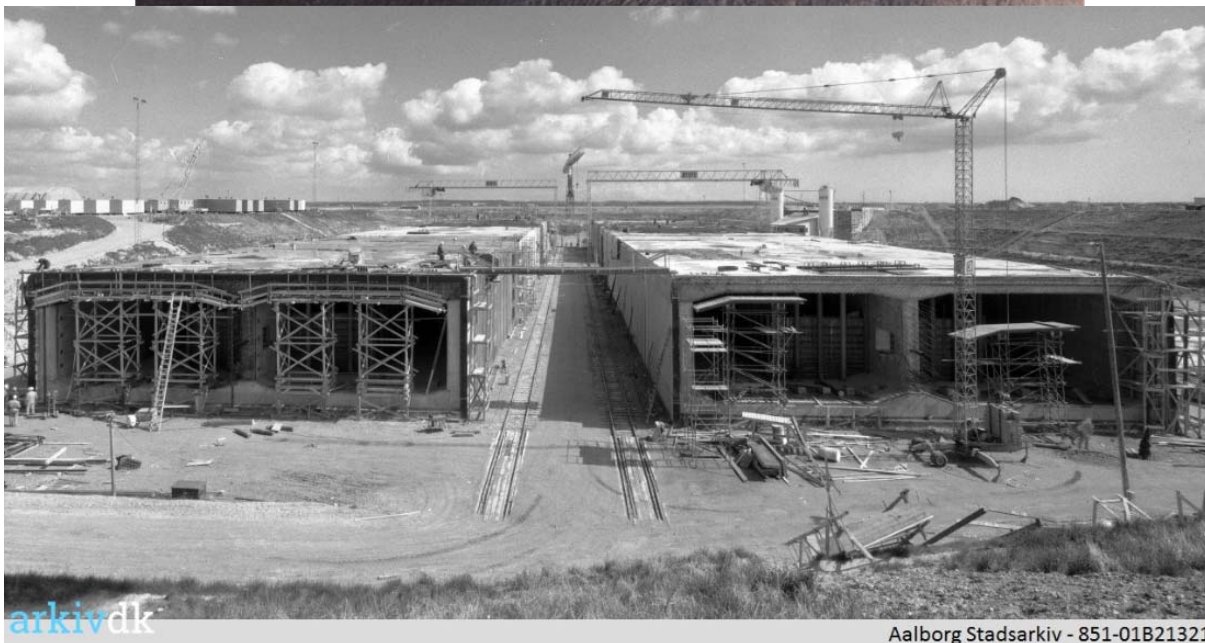
Figure 4.3-6 Casting of tunnel elements in the dry dock. The casting sections and openings can be seen on top picture.
