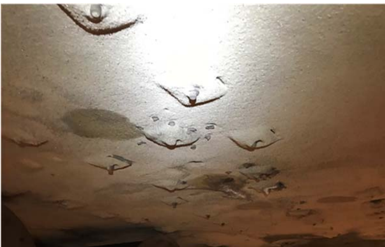
Figure 6.3-4 Area where fire protection has deteriorated.
