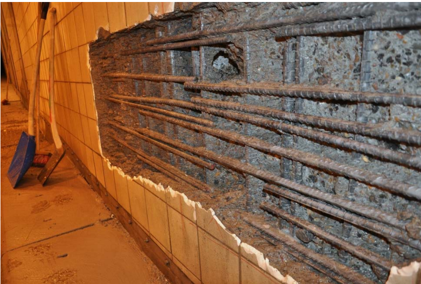
Figure 6.7-3 Exposed reinforcement at the closure joint (Type 2 joint). No signs of butt-welded connections in the horizontal reinforcement.
