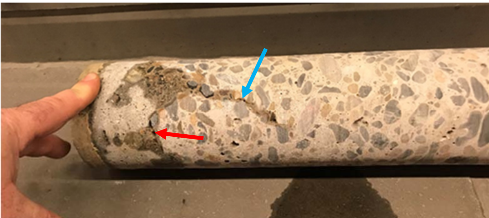
Figure 6.3-2 Core extracted from roof. The concrete is cracked both at the interface between repair and original concrete (red arrow) as well as within the original concrete (blue arrow).
